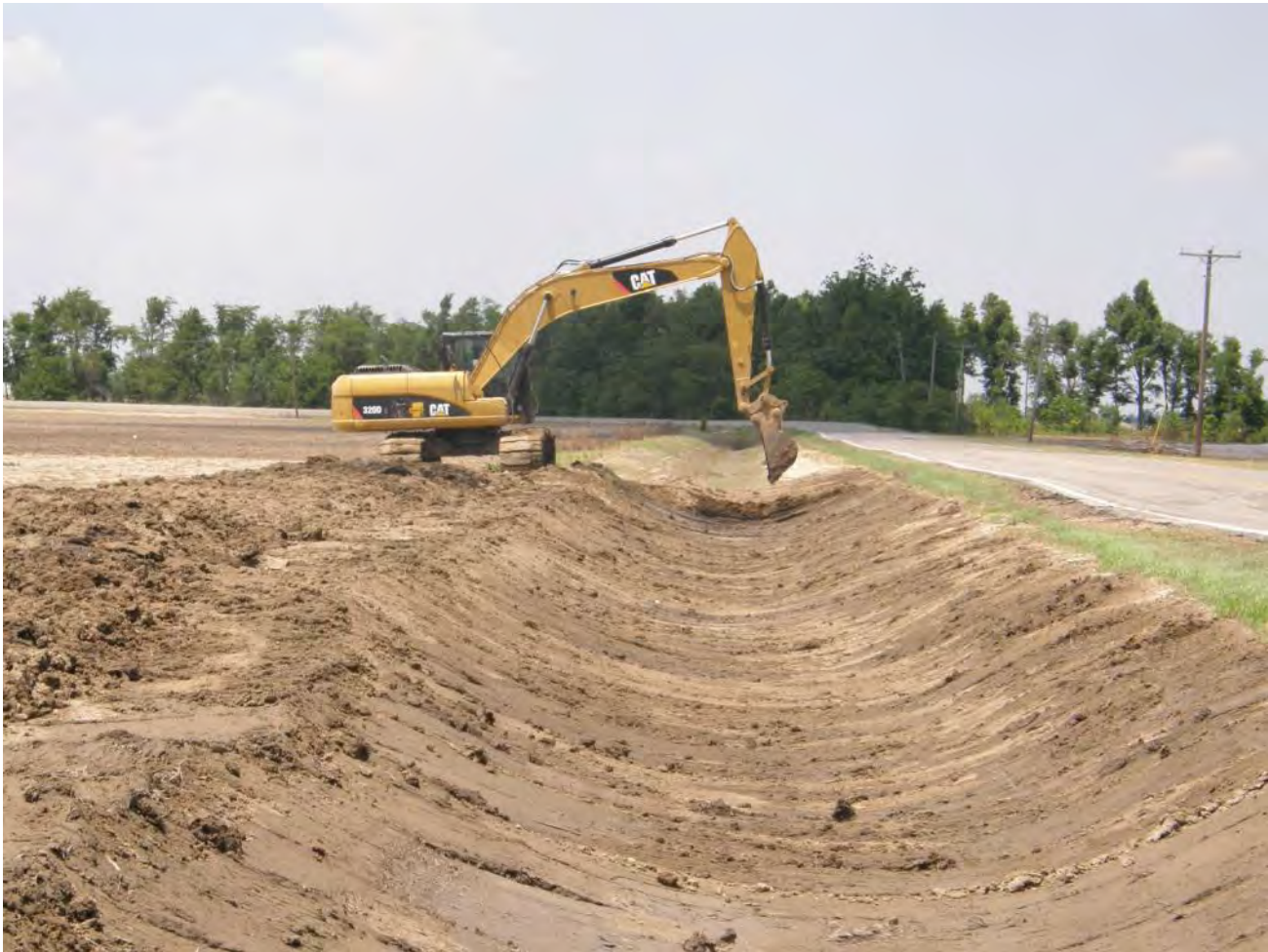
Figure 3. Silted in road ditch. Excavator cleaning out 2 feet of sediment in road and drainage ditches.
