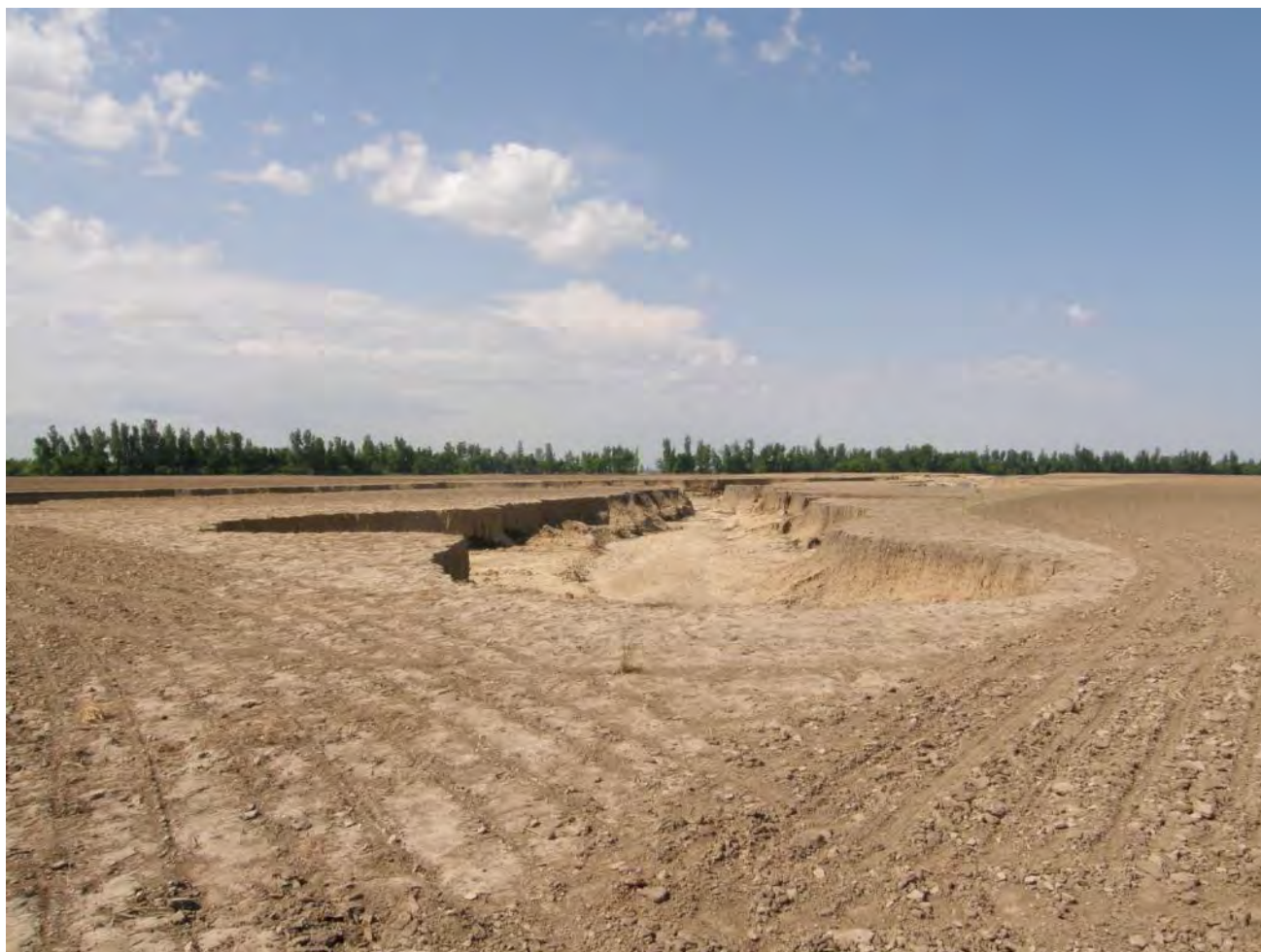
Figure 4. Field gullies in cropland. Gullies extended into cropland. Gullies and channels that was created from May 4-16, 2011. The main channel and attached gullies were up 8 to 12 ft deep and more than half of dissected field could not be cultivated.
