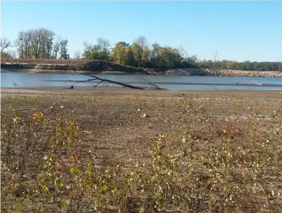
Figure 4. Breached levee. This breach occurred in January 2016 and is about one mile in length. Rip rap to the right of the levee breach was subsequently placed as a “repair”, but only covers a portion of the breach.
