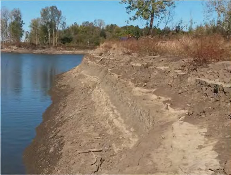
Figure 2. Sidewall of recently-incised channel through floodplain sediments at the Dogtooth Bend peninsula. The channel was formed as a result of a levee breach in January 2016. The breach was still open on the tour date and the nearly 7,000-foot long channel still connected to the Mississippi River. Dr. Olson pointed out that subsequent flood events may lengthen the channel and cause more damage. Ultimately, it could enter an older meander scar and re-connect with the river, making the peninsula an island.
