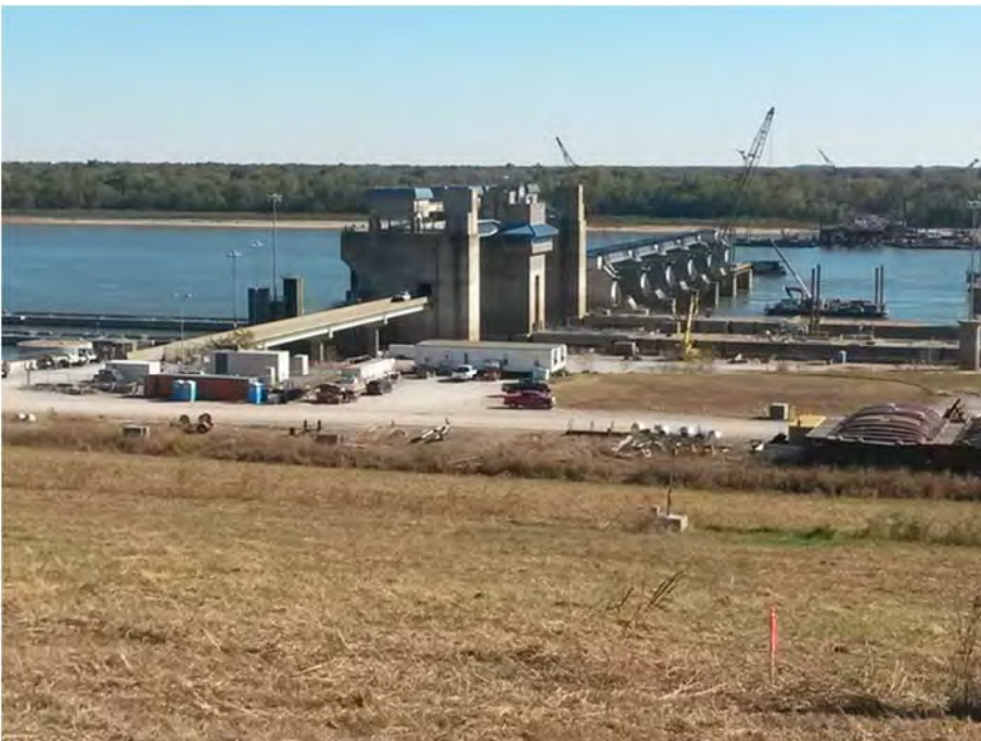
Figure 5. The Olmstead Lock and Dam on the Ohio River. This $2.9 billion project was started in 1995 and is scheduled for a 2020 opening. Completion of this structure along with the removal of two sets of locks and dams upstream will reduce navigation time on the lower Ohio River by 3 hours.
